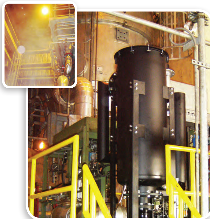
Alstom GT11NM Gas Turbine Inset: Hazardous Oil Mist Emissions from Previous Electrostatic Precipitator. After: Clean and Safe Work Environment with a Oil Mist Eliminator.
